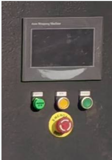
Control detail | Operator panel and emergency stop
